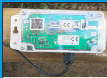
Micro controller radio sensor unit on FRP Pipeline
